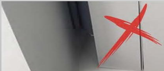
Unlevel and out of square corners
