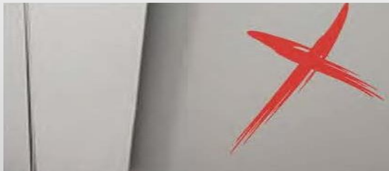
Uneven gaps from wavy drywall
